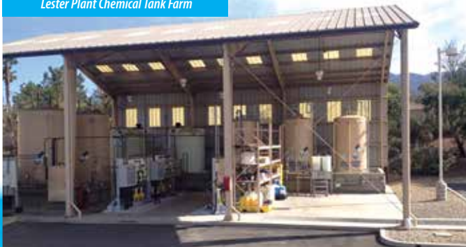
Lester Plant Chemical Tank Farm
